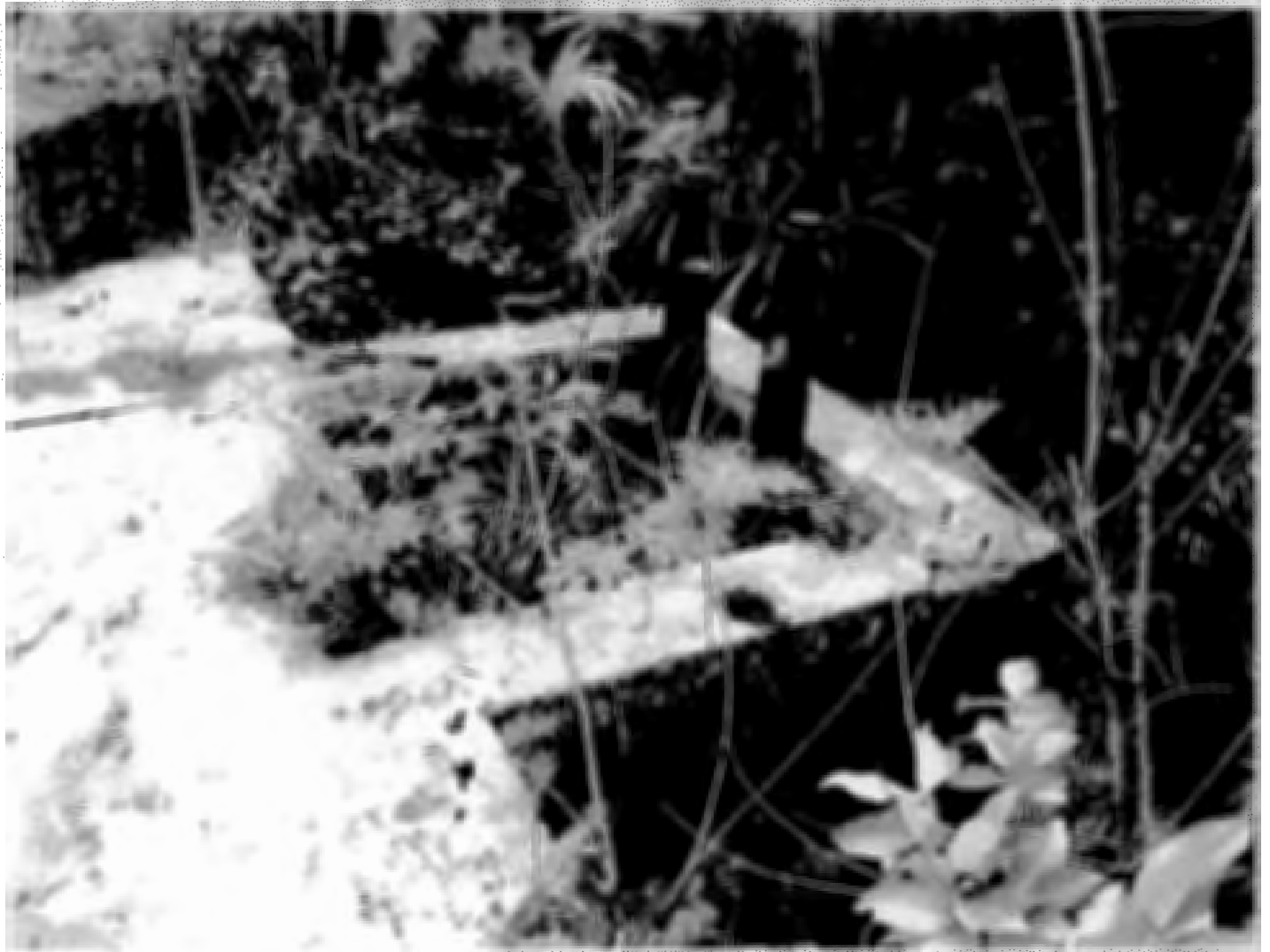
Figure 4: View of the two valves labeled Chapman Valves / C (over) V MFG. CO. / Boston / U. S. A.
